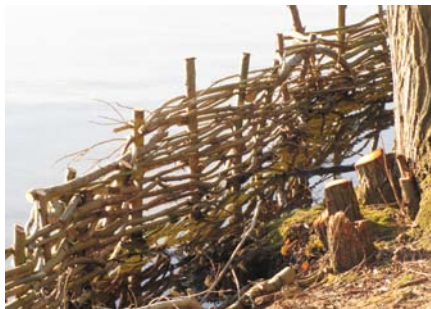
3. Willow branches woven to create a natural fence that removes wave energy.
