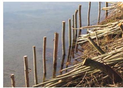
2. Willow stakes driven into the lake bed where the bank is threatened by erosion from wave action.
